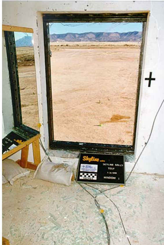
Interior view of glass fragments inside the reaction structure.
